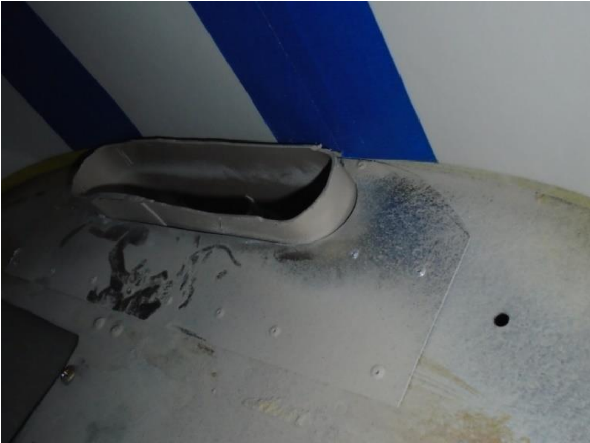
Figure 2 – AC-02560 Evaporator Outlet Trimmed Down
