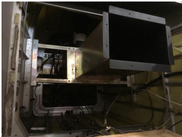
Figure 12 - Cabin Inlet Duct
