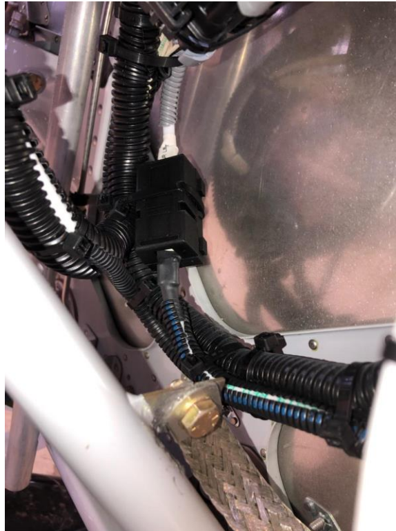
Figure 14 – 70 Amp Fuse Approximate location of 70 Amp fuse located below Lamar Electrical Junction Box on Firewall
