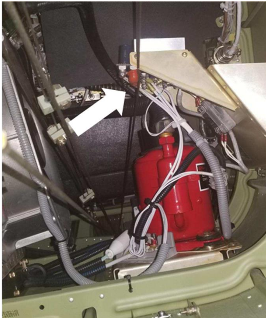
Figure 1 Improper Routing of Rudder Cable Rudder cable is caught between mounting bracket and power stud on circuit board.
